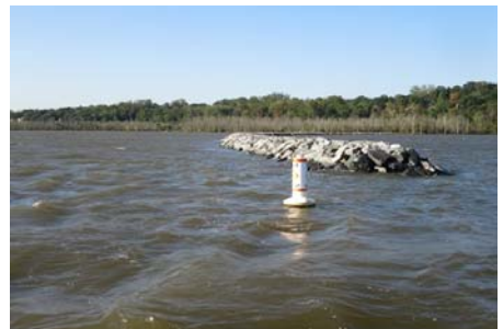
The breakwater, which replicates the removed protective promontory, is nearing completion. Photo by Glenda Booth
