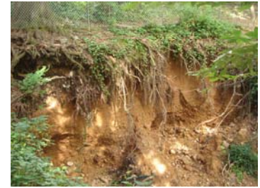
The gouged out stormwater outfall in Mt. Vernon Park.
