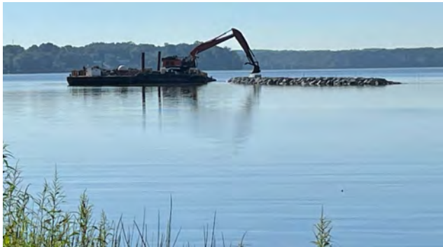
A barge places rocks on a new sill. Photo by Dorothy McManus
