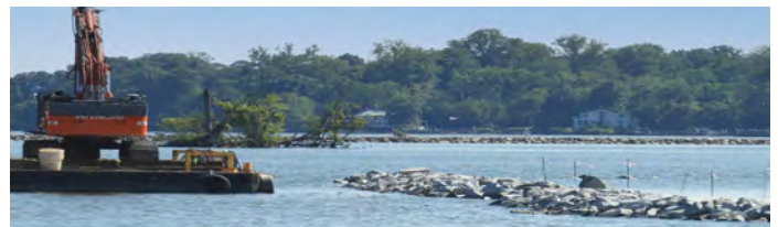
Barge and new sill in foreground with older sill in the distance Photo by Bob Veltkamp
