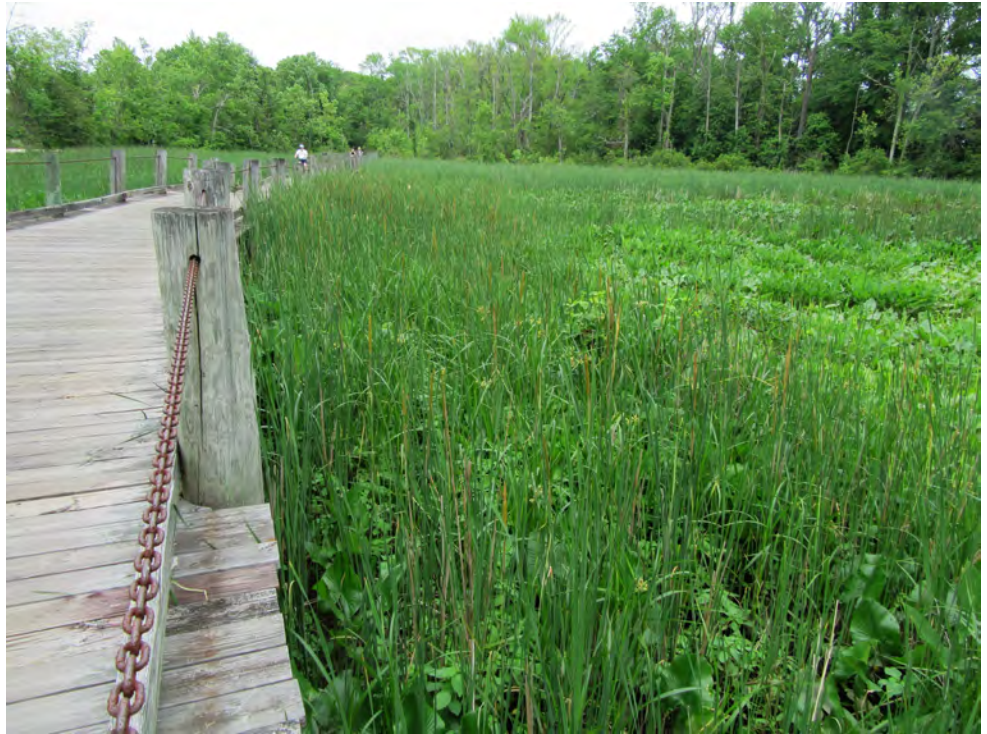
The bridge spans the wetland, giving people an up-close view of the diverse plant life of Dyke Marsh.
